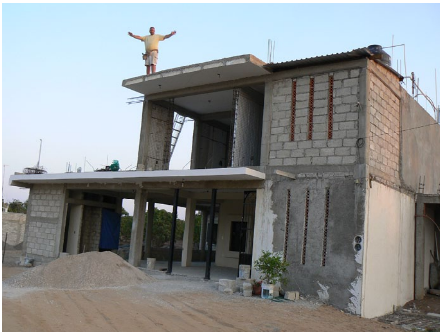
Phil Shirey came down and helped with wiring and plumbing. Thanks Phil!!
