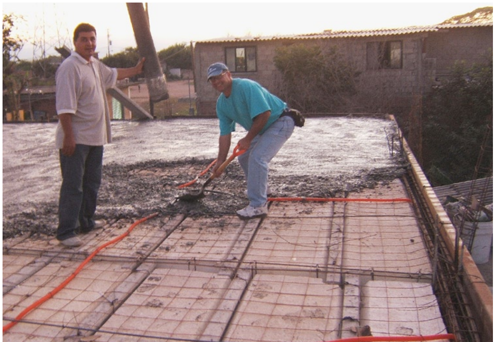
Pastor Luis Miguel and Lee pose for the camera during the roof pouring.
