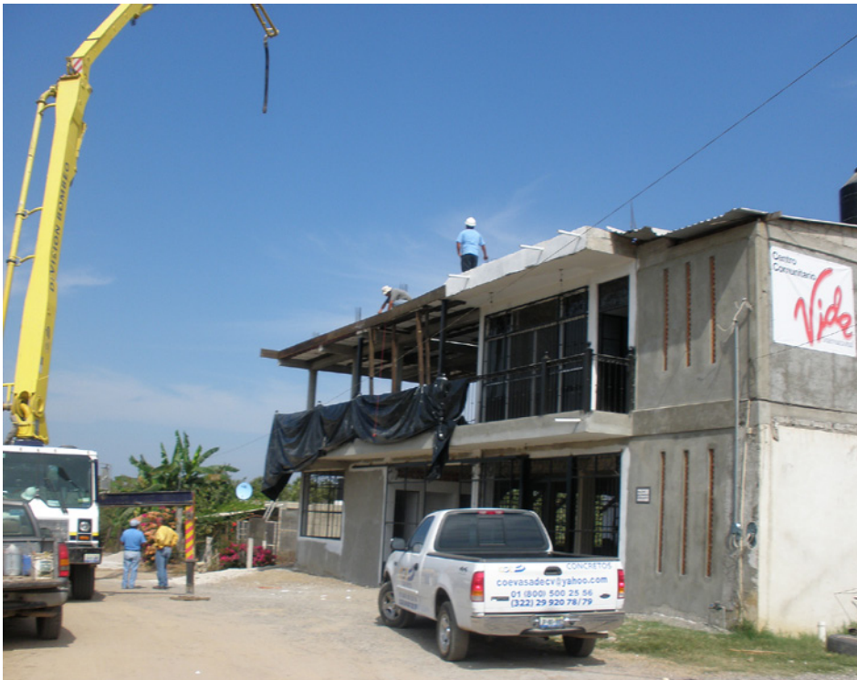
Pouring the roof for the ministry office, windows and walls still needed!
