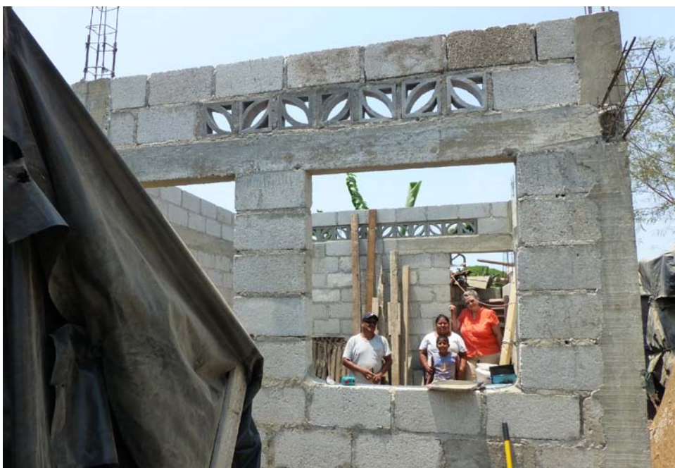
Progress on Emiliano’s house. This is two rooms. Next a roof, then two more rooms.
