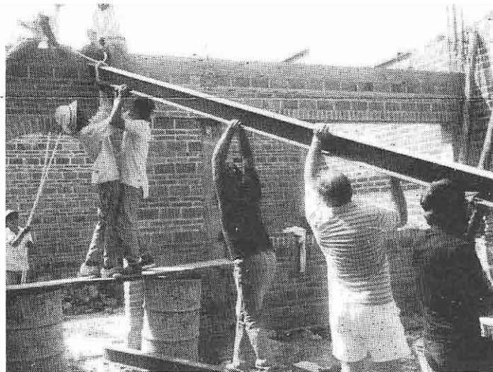
Lifting "I" beams by hand. Lee and his dad inside the video studios.
